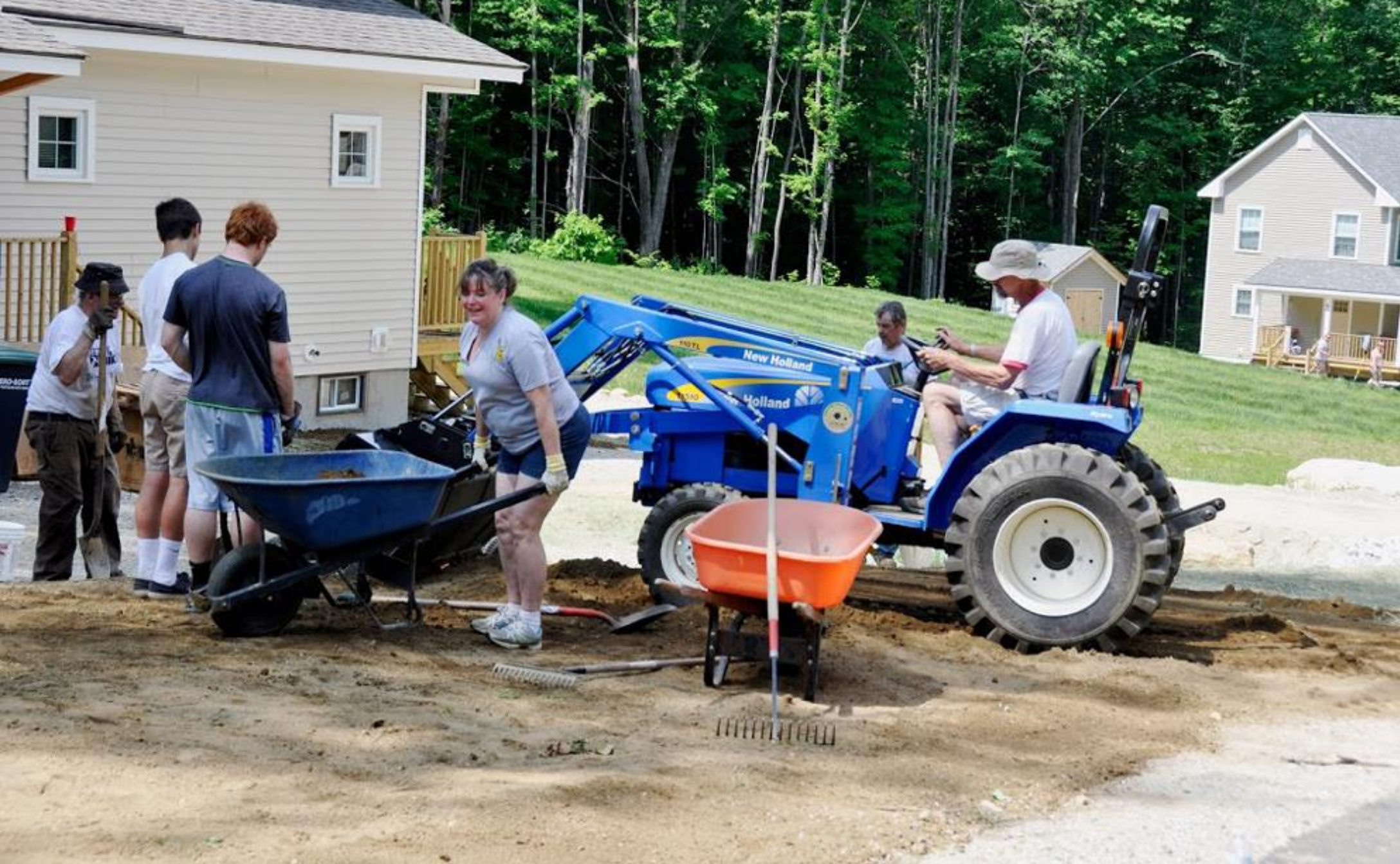
On Jennifer Lane in Manchester, Bennington Habitat for Humanity is developing a new neighborhood with a total of 22 lots designated by Town Permit for affordable housing.
