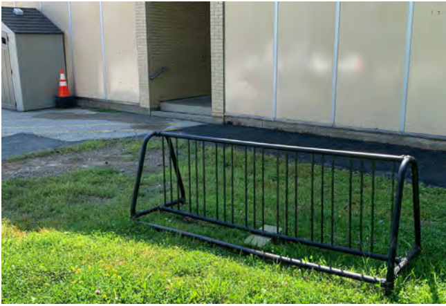
Monument Elementary's bike rack does not allow locking of the frame and can cause front wheel damage.
