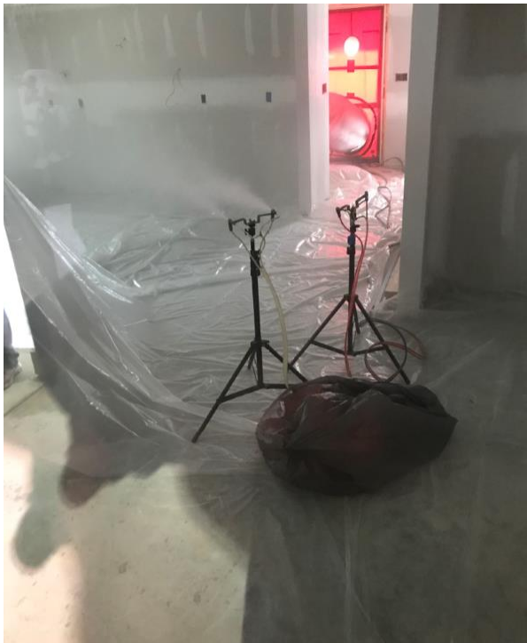
Aerobarrier sealing in progress. The red “door” is the “blower door” sealed in the door opening with a fan which pressurizes the building (apartment) during installation.
