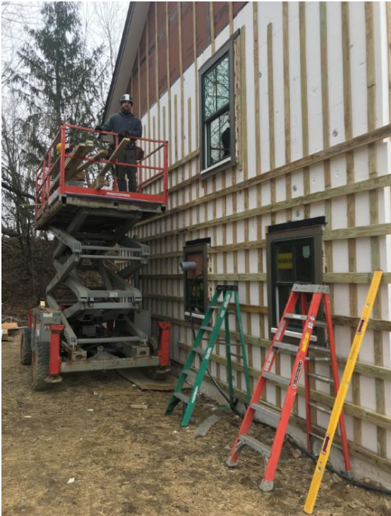
3" of EPS (expanded polystyrene) continuous insulation installed to the exteriors of the buildings and strapped for siding installation. EPS was selected for the relatively low GWP of the blowing agent used for its manufacture.
