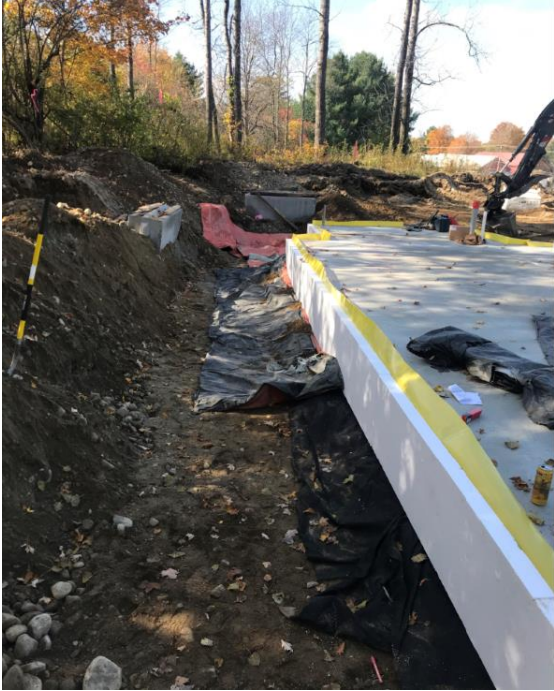
FPSF slab has been poured and slab edge insulation is installed. The vapor barrier protruding above the slab will be taped to the sheathing to maintain continuity of air barrier.
