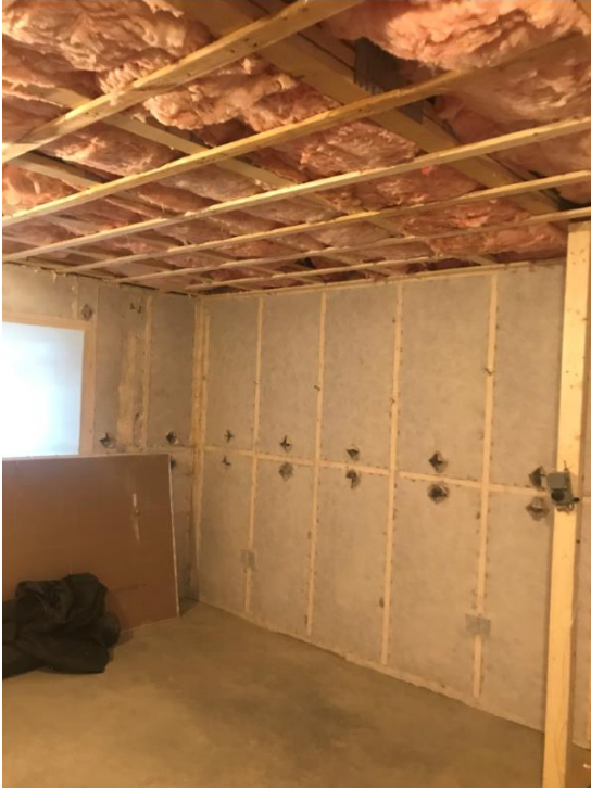
Densepacked cellulose insulation installed in exterior and demising walls. The pink fiberglass batts provide sound insulation in floor/ceiling assemblies.
