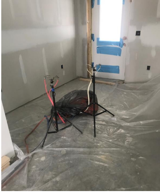
Aero Barrier emitters prepared for spraying acrylic aerosol caulk. Horizontal surfaces are protected from caulk that will settle from air.
